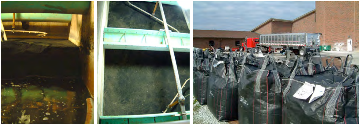
18" GAC Filter Cap - Bloomington, Illinois; Replacement of GAC media (in black totes)
