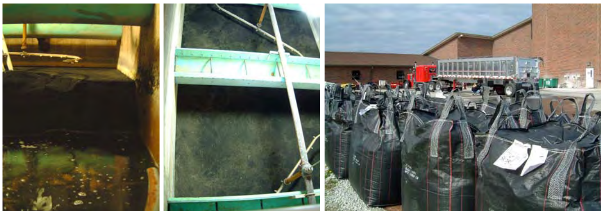
18" GAC Filter Caps - replacement of GAC media (virgin GAC in black totes)
